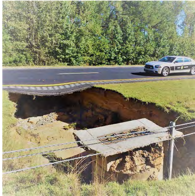
FIGURE 5.12: SINKHOLE IN NORTH CAROLINA
