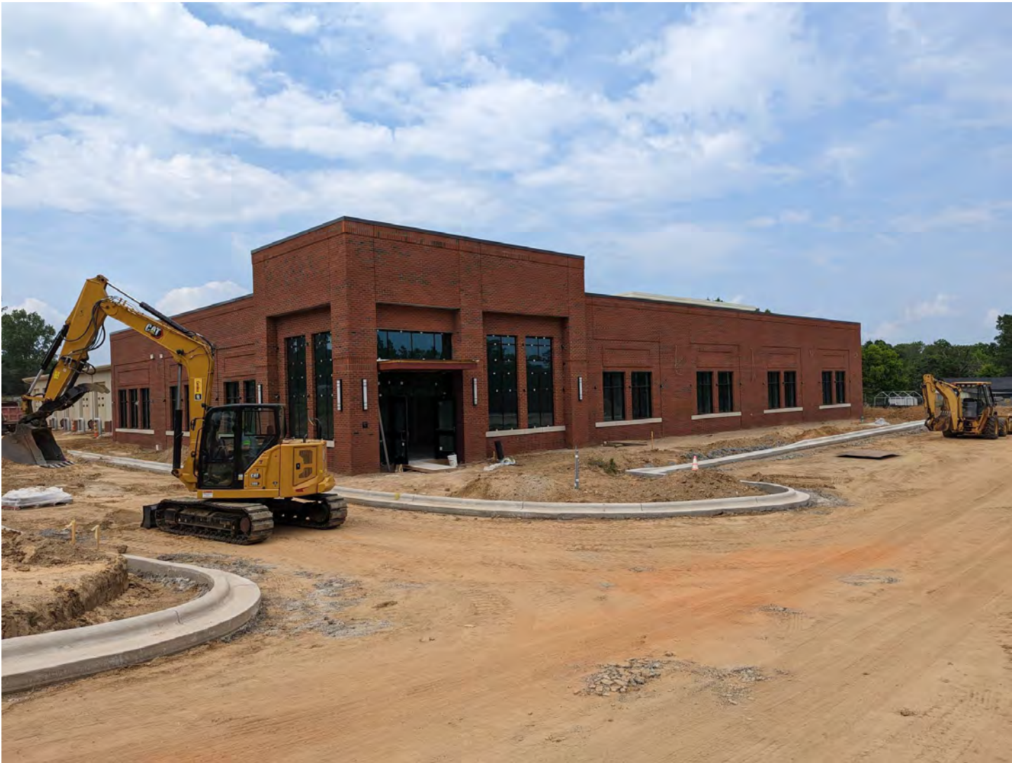
View of front entrance to ITS from the entrance off of Ramdin Ct.
