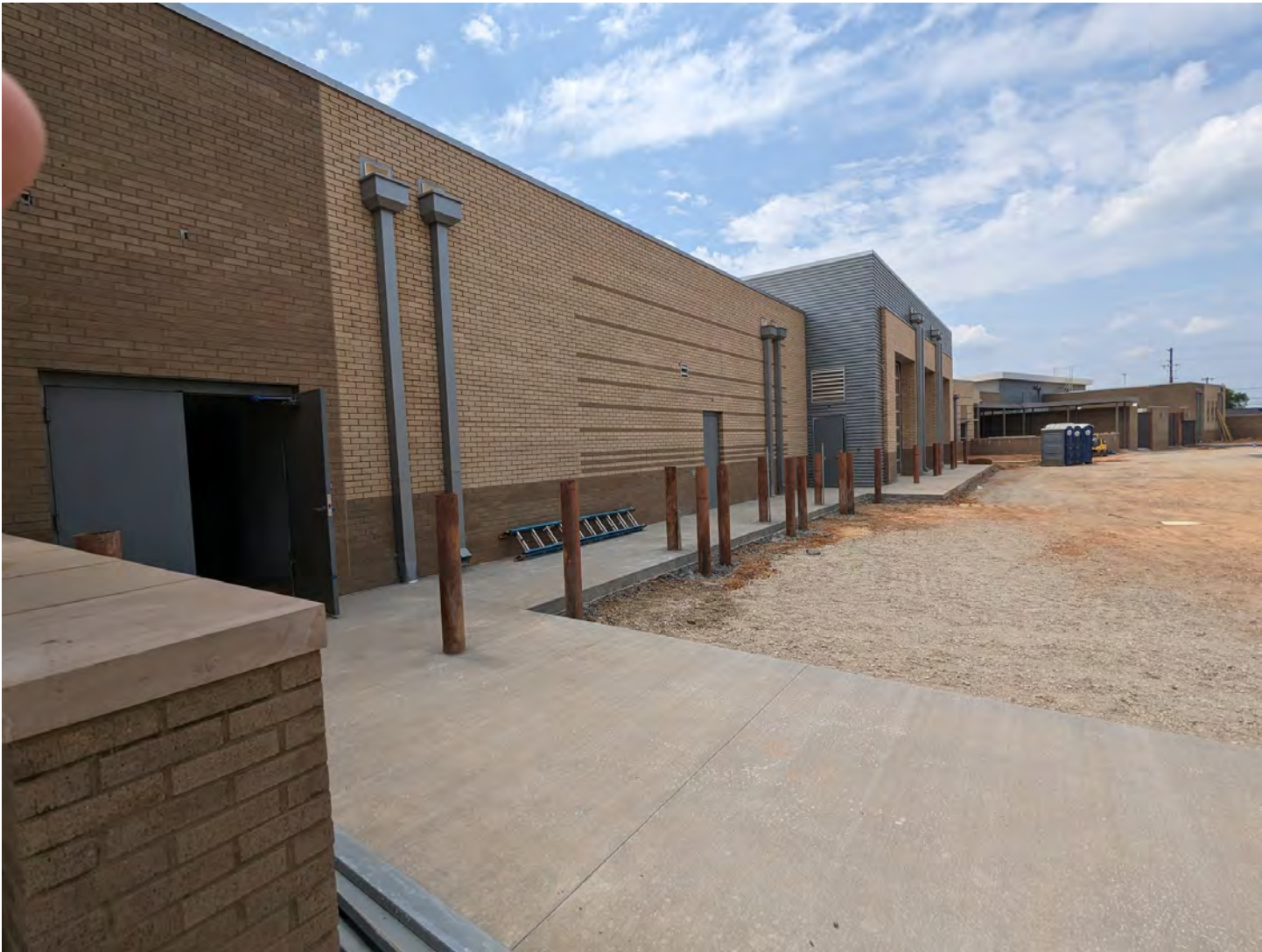
Back side of the building outside of Medical Supply Storage and the Delivery Vestibule
