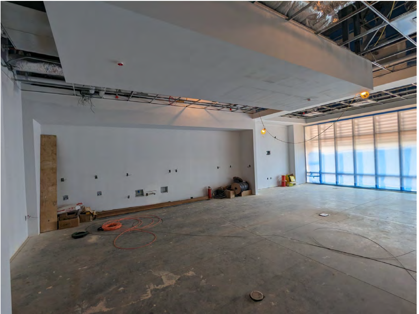
This is the Kitchen/Dining Room on the left side of the picture and the Dayroom on the right side of the picture
