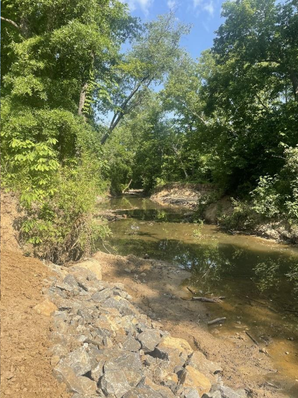
After debris removal
